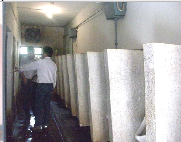
Gents toilet block with lighting and exhaust fan
