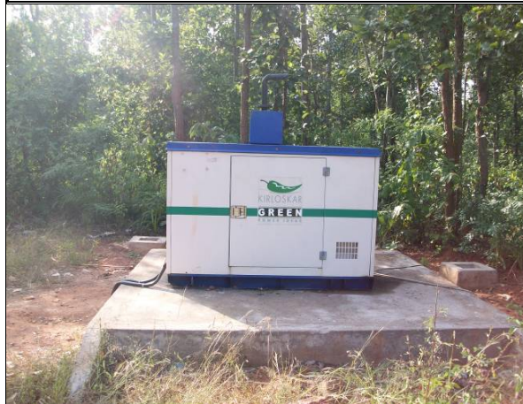
Green Generator with acoustic sound enclosure
