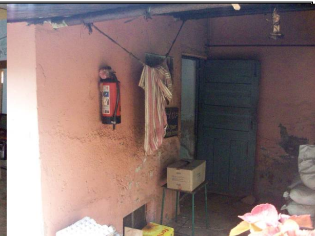
Fire extinguisher outside LPG store room
