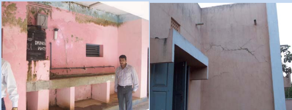
The above pictures damp affecting electrical wiring at Jawahar Navodaya Vidyalaya and cracks hostel building of Government Girls High School (Girls), Dutipada respectively
