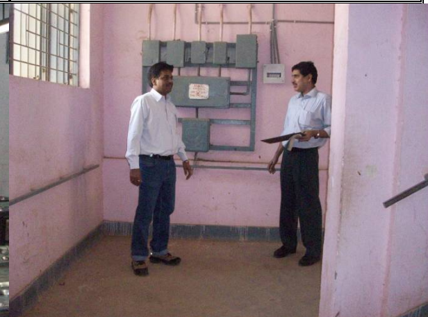
Main switch at very low height behind the staircase
