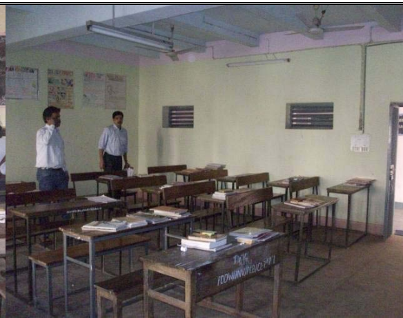
Ventilators for cross ventilation at the classroom
